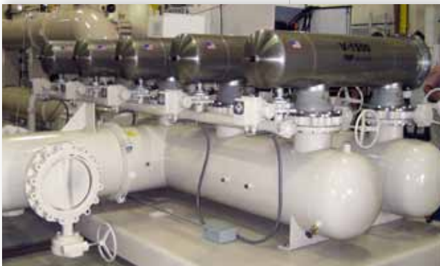
The pump station was custom-engineered and performance-tested, as shown above, at the Watertronics facility in Hartland, Wisconsin, USA.
