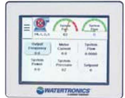
PLC controls offer intuitive touchscreen navigation
